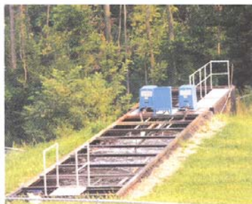
Package plant installed below ground. Control panel and modular blower package are shown.
